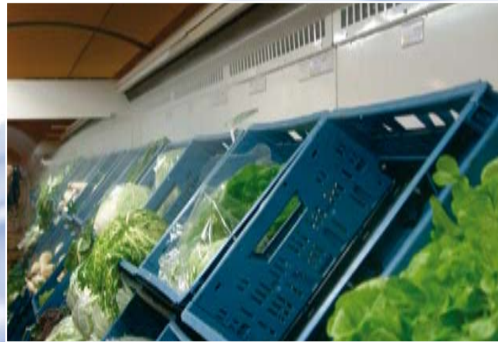
In the professional ultrasonic humidifying system an aerosol mist formed of tiny water droplets is captured by the current of cold air and drifts around and through the fresh produce, preserving its quality.
